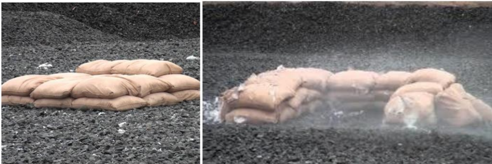
Figures 4 and 5: Example of a Sandbag Backstop before and after demolition (Reference: google website)
